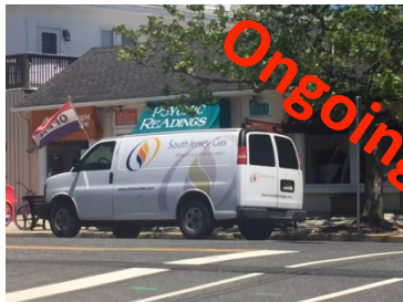
SJ Gas Upgrades
